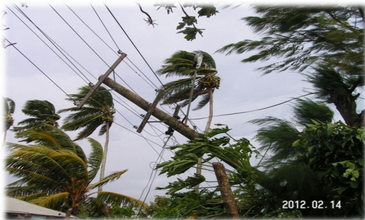
Fig 5: Broken Poles as a result of cyclone Jasmine
